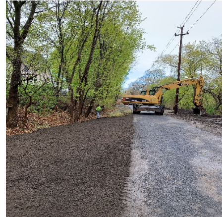
RZC spreading loam at trail shoulders from Central St. to Denver St.
