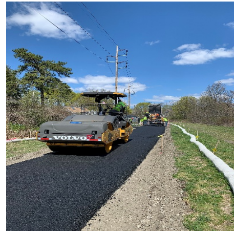
BROX installing Superpave Intermediate Course between Salem St. & Lynn St. (Sta.139+42 - Sta.100+50).
