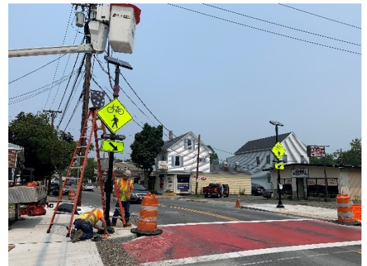
Pine Ridge.: installing Rectangular Rapid Flashing Beacon pole assembly at Central Street in Saugus.
