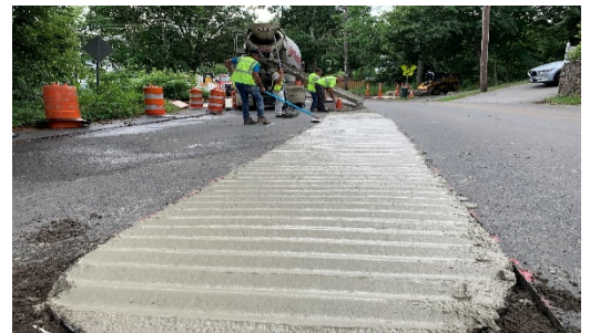
K. DaPonte Conc. pouring concrete for Scored Cement Median at Adams Ave.
