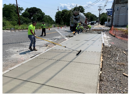
K. DaPonte Conc. pouring concrete for sidewalks and WCR at Salem Street in Revere
