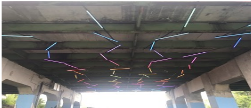
Pine Ridge activated lighting under Route 99 overpass in Revere.
