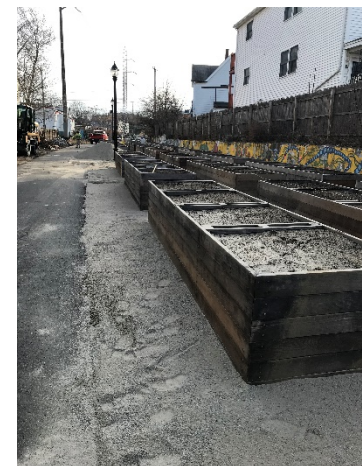
RZC installing Raised Garden Planter beds at West Street Community Garden, Everett.
