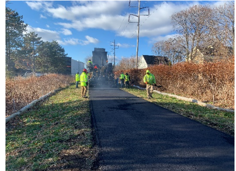
BROX installing Superpave Surface Course for Bike Path between Bocce Court and Lynn Street, Revere
